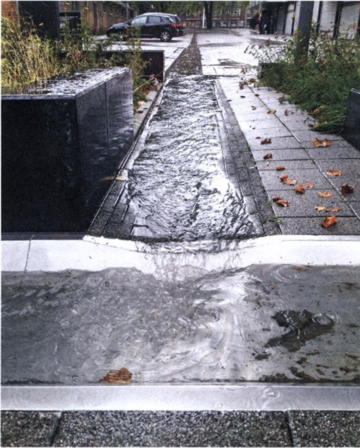
Waterdrain via specially designed gutters.
