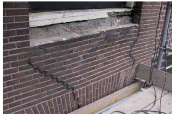
Subsidence as a result of drought
