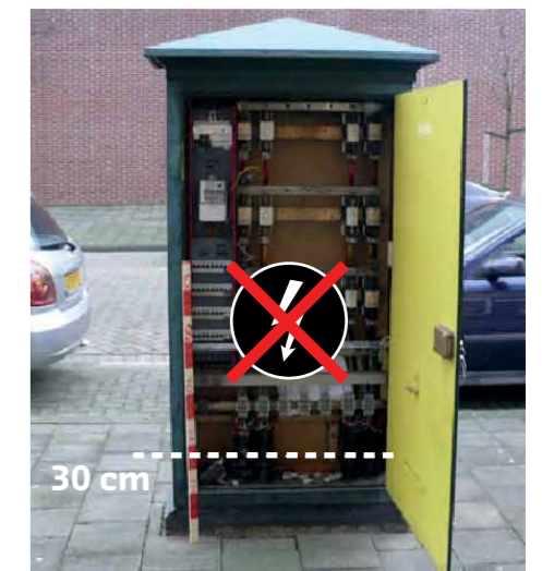
Transformer stations are vulnerable to inundation depths greater than 30 cm
