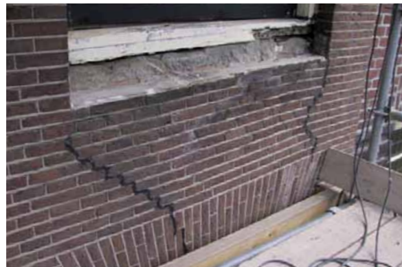
Subsidence as a result of drought
